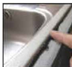
Caulking eventually becomes dislodged creating a recurring maintenance issue
