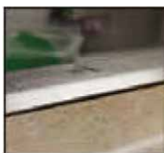
Gap between the countertop and the sink rim causes water seepage
