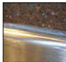
Unsightly caulking needs constant maintenance
