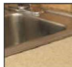
Sink rim creates a ridge that makes it difficult to clean
