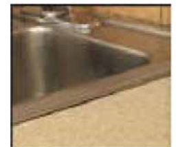
Sink rim creates a ridge that makes it difficult to clean
