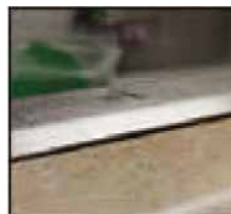
Gap between the countertop and the sink rim causes water seepage
