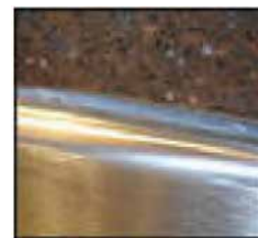
Unsightly caulking needs constant maintenance
