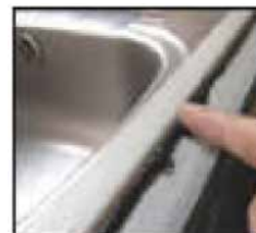
Caulking eventually becomes dislodged creating a recurring maintenance issue
